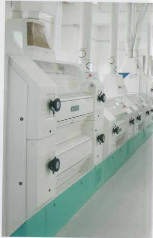
The roller floor boasts a total of thirteen four-roller mills (MDDM) and two eight-roller mills (MDDO).
