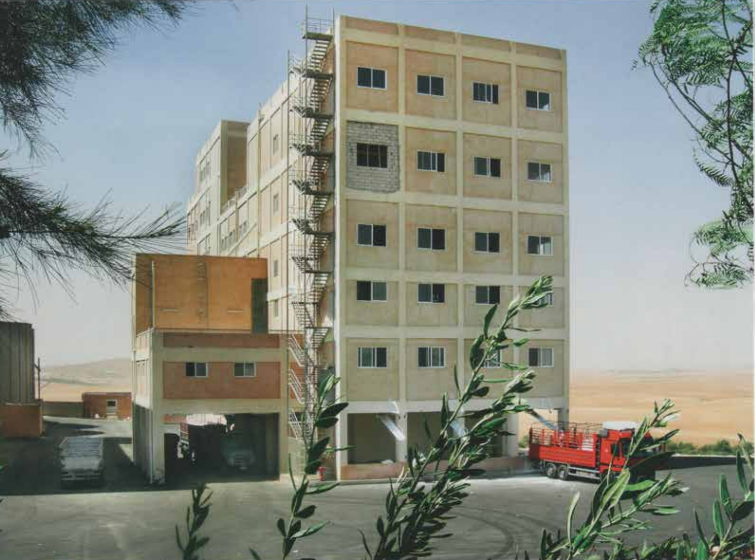
The new 320-ton flour mill of South Amman Mills in Amman.
